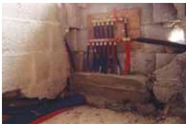
Hot and Cold Water Supply Distributors, installed in a Cabinet
